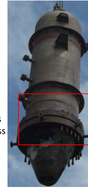
Usual damaged heat exchanger localization
